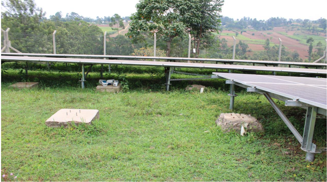
Solar panels installed at the Powerhive project, Miwani village.
